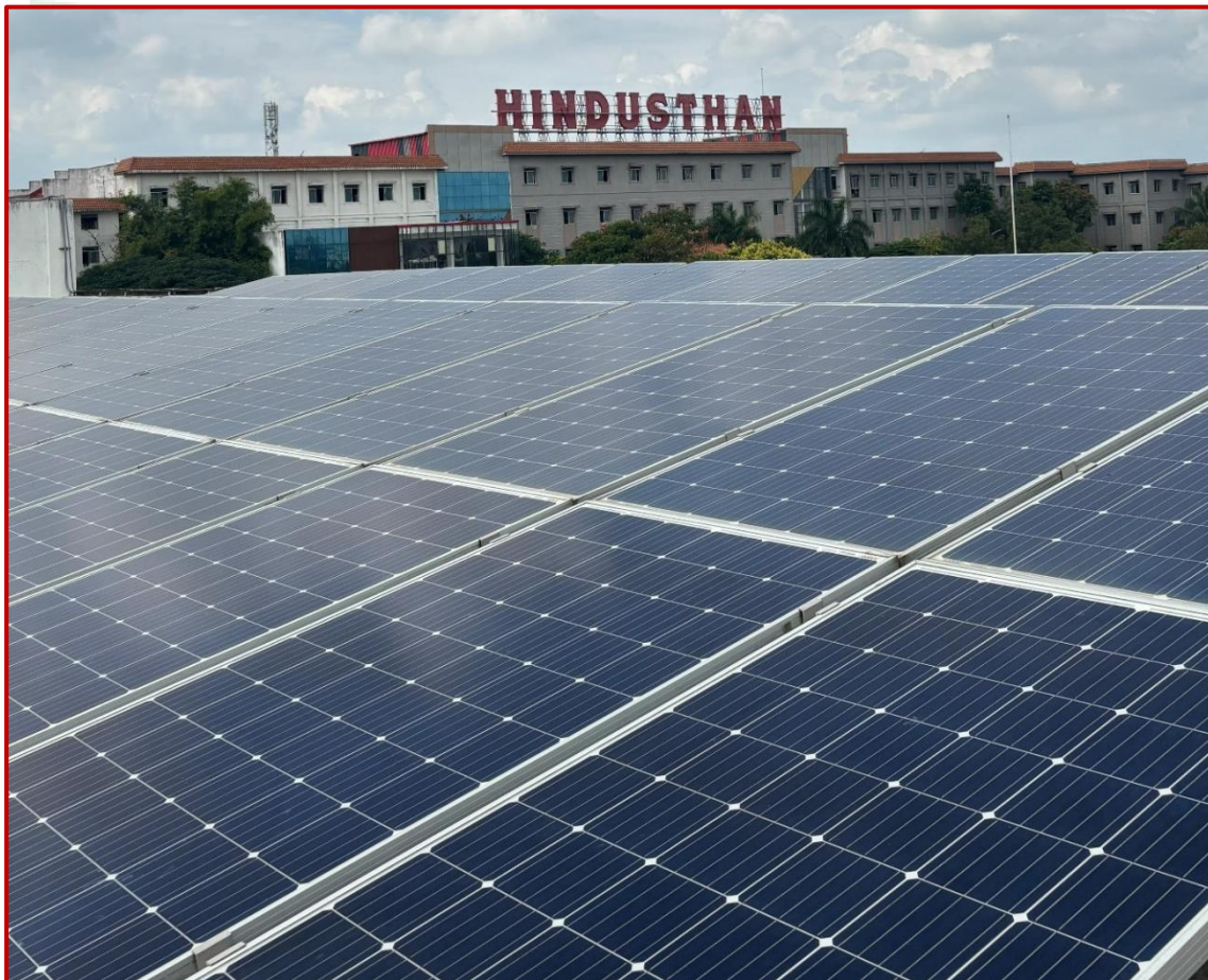
Solar PV Plant
