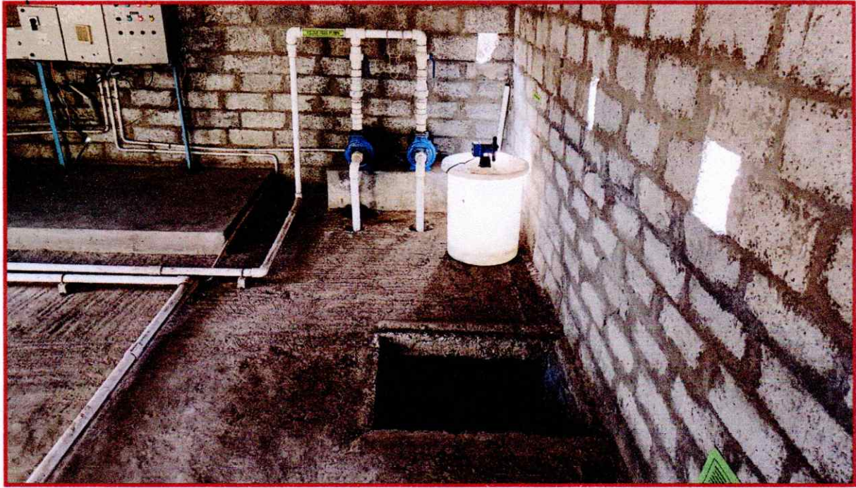
Figure 8 Filter Feed Tank (Capacity 40KLD) & Filter Feed Pump
