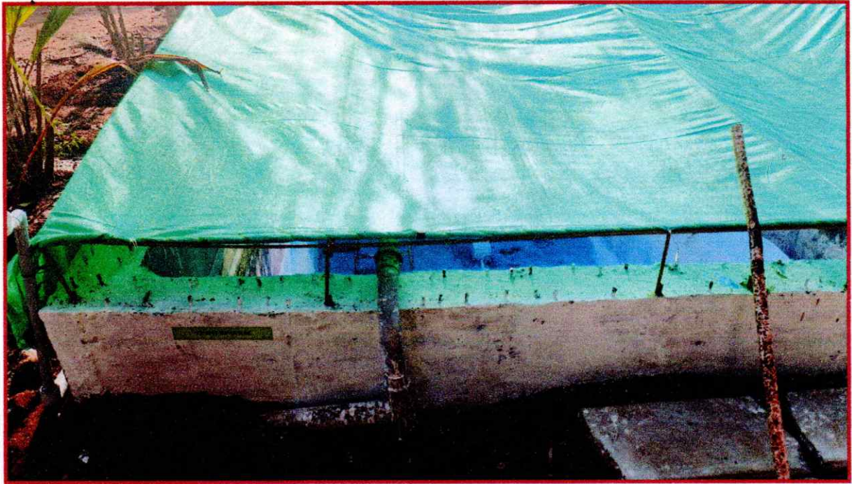
Figure 10 Treated Water Tank (Capacity 100KLD)
