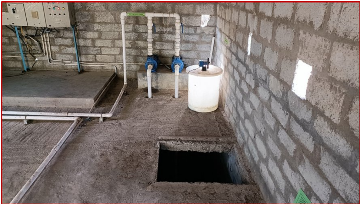
Fig. 4.7 Filter Feed Tank (Capacity 40KL) and Filter Feed Pump
