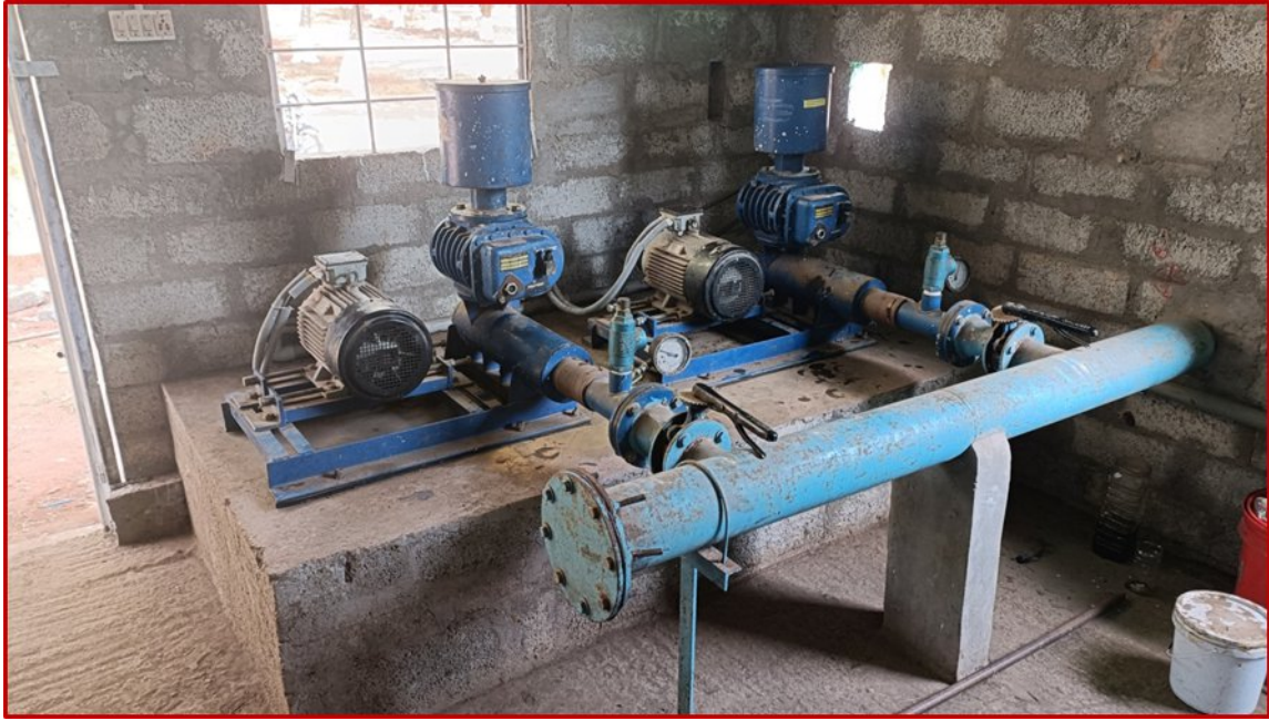
Fig. 4.6 Air Blowers for Aeration
