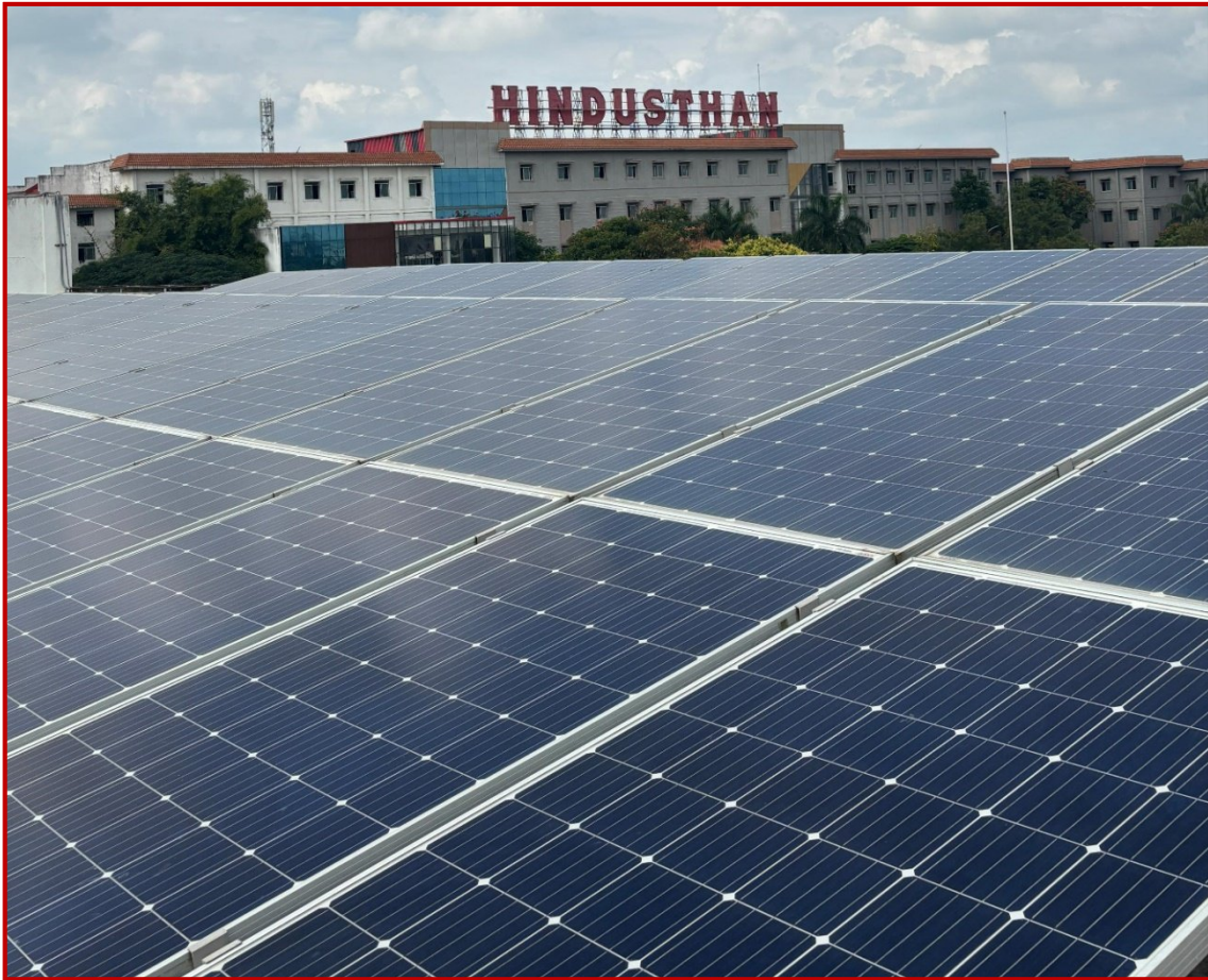
Fig. 3.1 Solar PV Plant
